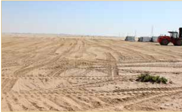
Work at the Sertun Energy Plant - Trekkopje - Erongo Region (Solar).
