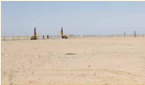
Work at the Sertun Energy Plant - Trekkopje - Erongo Region (Solar).
